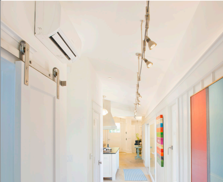
O'Neill Passive House, Wall-mounted Unit
