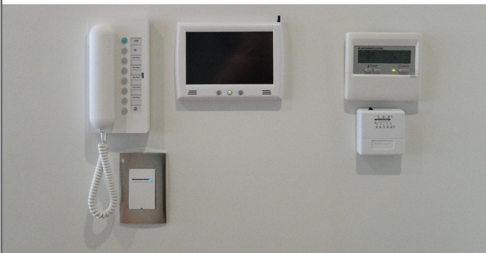
Novogratz House, New York City, N.Y. Ceiling-cassette Unit Controller
